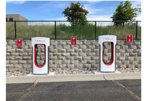
BATTERIES AND EVS
