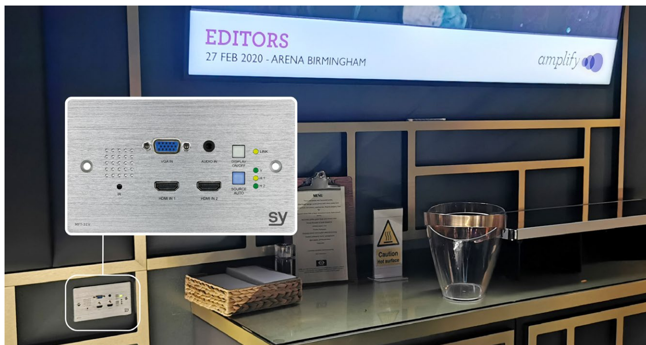
NEC VIP Suite SY Electronics MFT-31V multi-format input plate with TV monitor display control and HDMI and VGA inputs, which sends the signals to the display via HDBaseT.
